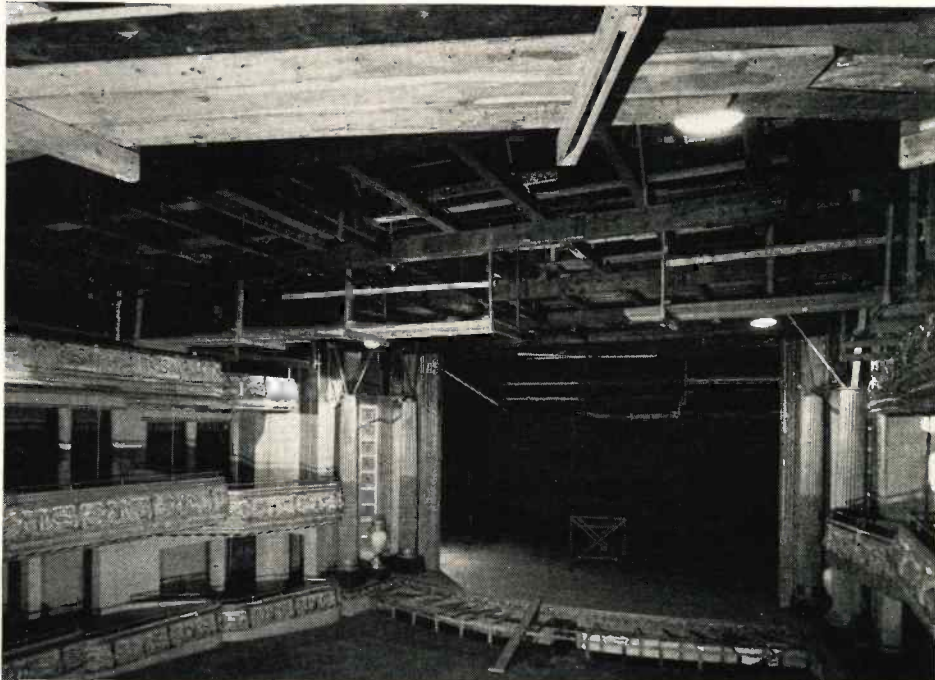
Hollywood's conversion to television continues as ABC video takes over this Warner Brothers sound stage along with other buildings on the 20-acre site.
